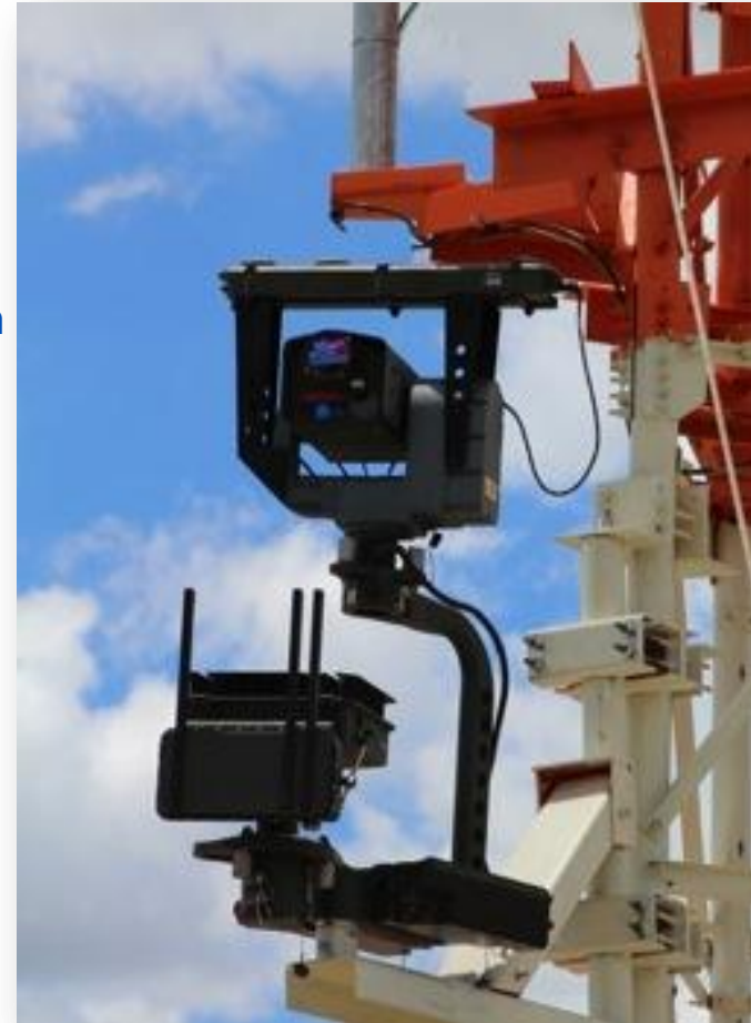
Radar and Cameras integrated at tower
